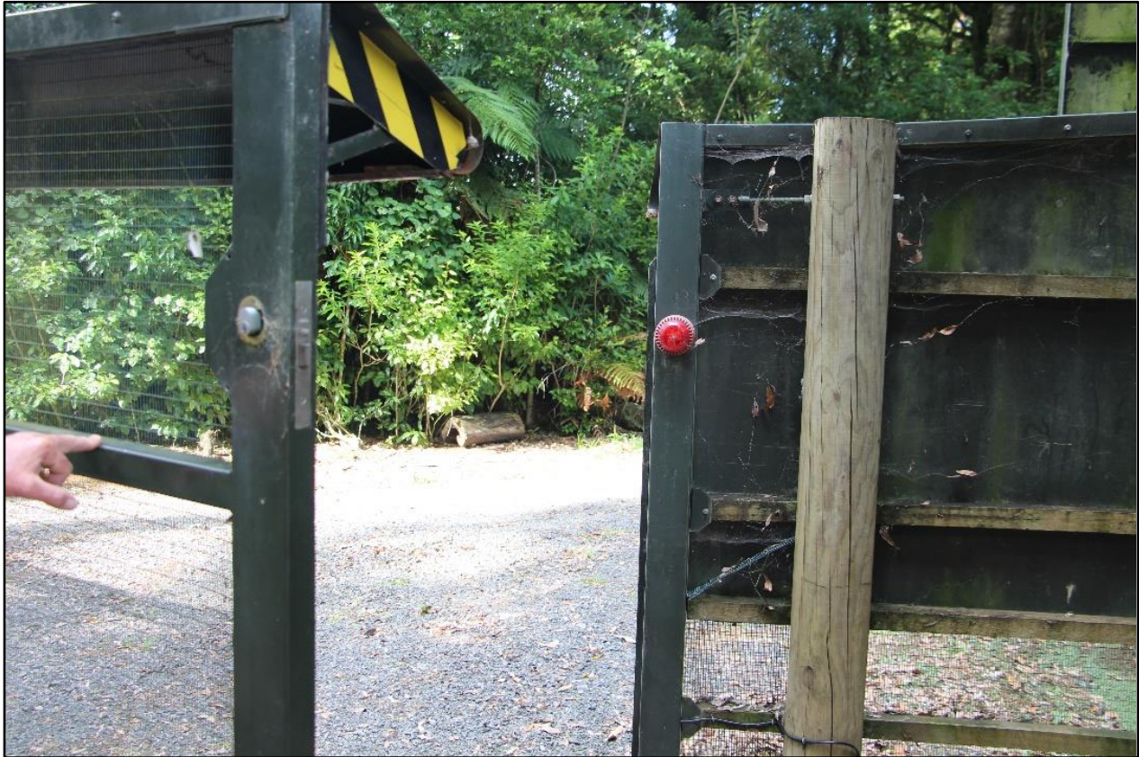
Figure 7: A vehicle gate showing the upper slam lock and red warning light
