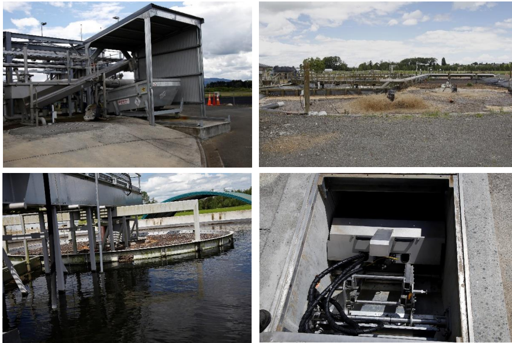
Figure 2 - Major improvements from left clockwise include the inlet works modifications, aerator addition, UV reactor system upgrade, and additional clarifiers.
