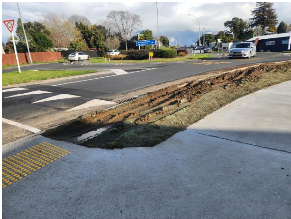
Figure 12: Wheel Tracks Observed at Northwestern Corner of the Roundabout
