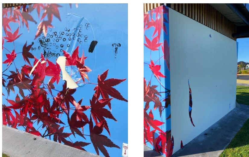
Damage to the wall wrap at Terry Came Drive, Cambridge
