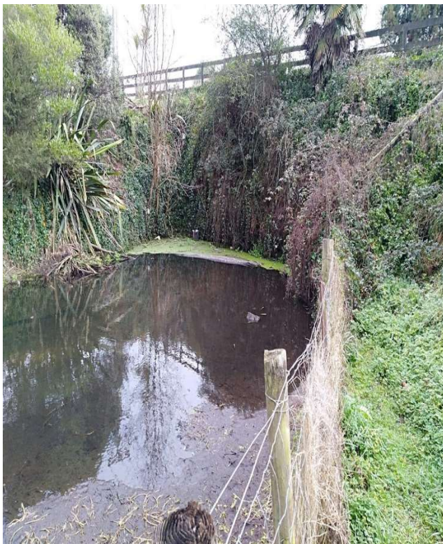
Photo 7: Submerged Culvert Inlet Under Cambridge Road
