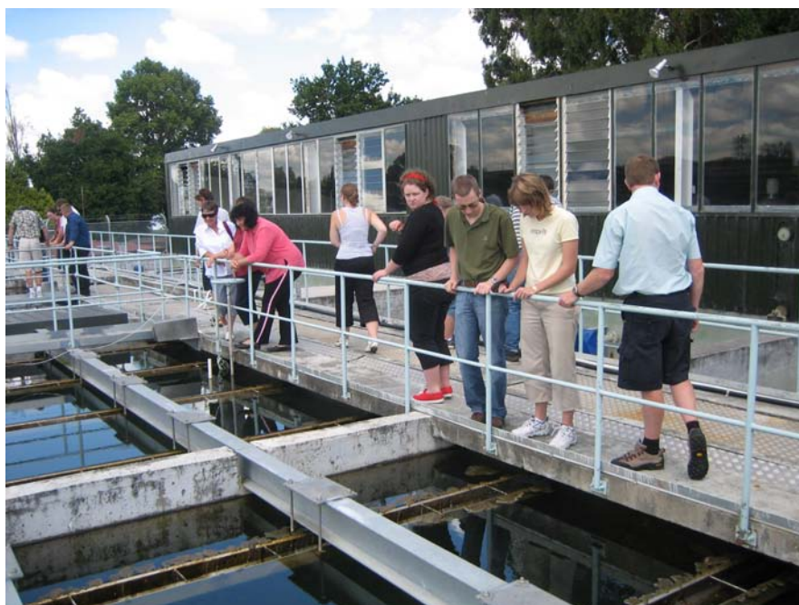
Karapiro Water Treatment Plant, Cambridge
