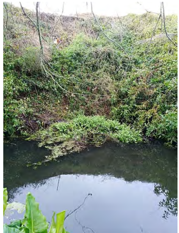
Photo 8: Submerged Culvert Outlet Under Cambridge Road
