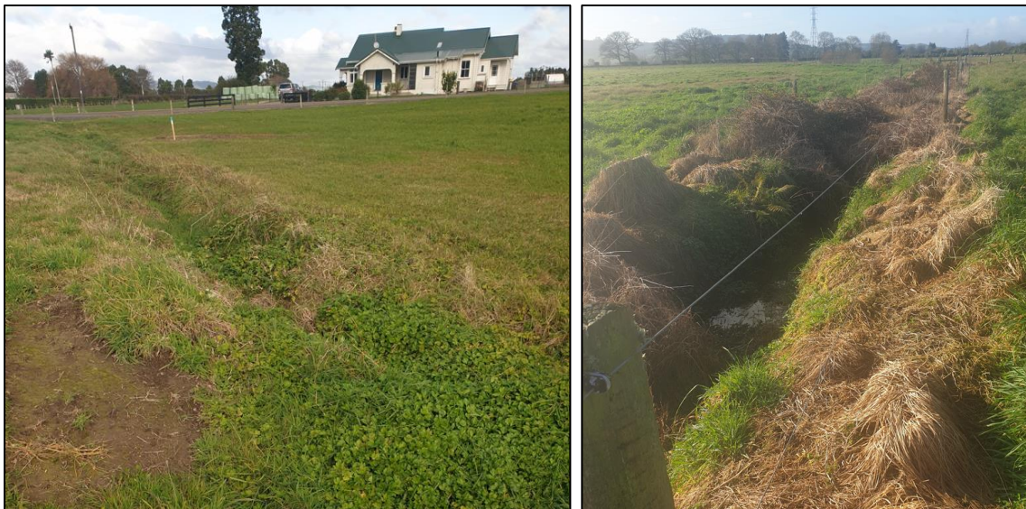
Figure 24: Images of cut drains, unmaintained to the left, and maintained to the right.
