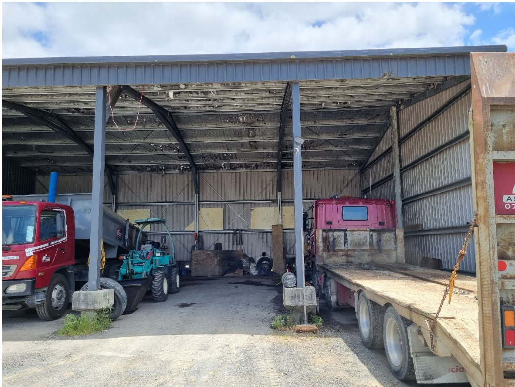
Photograph 22: 'Workshop' / Storage shed containing trucks, loader, digger and a Bitelli asphalt paver. Numerous stains on ground and general storage (i.e. empty 20L containers of engine/lube oil, tyres, carpet etc) (Feature of interest 15).
