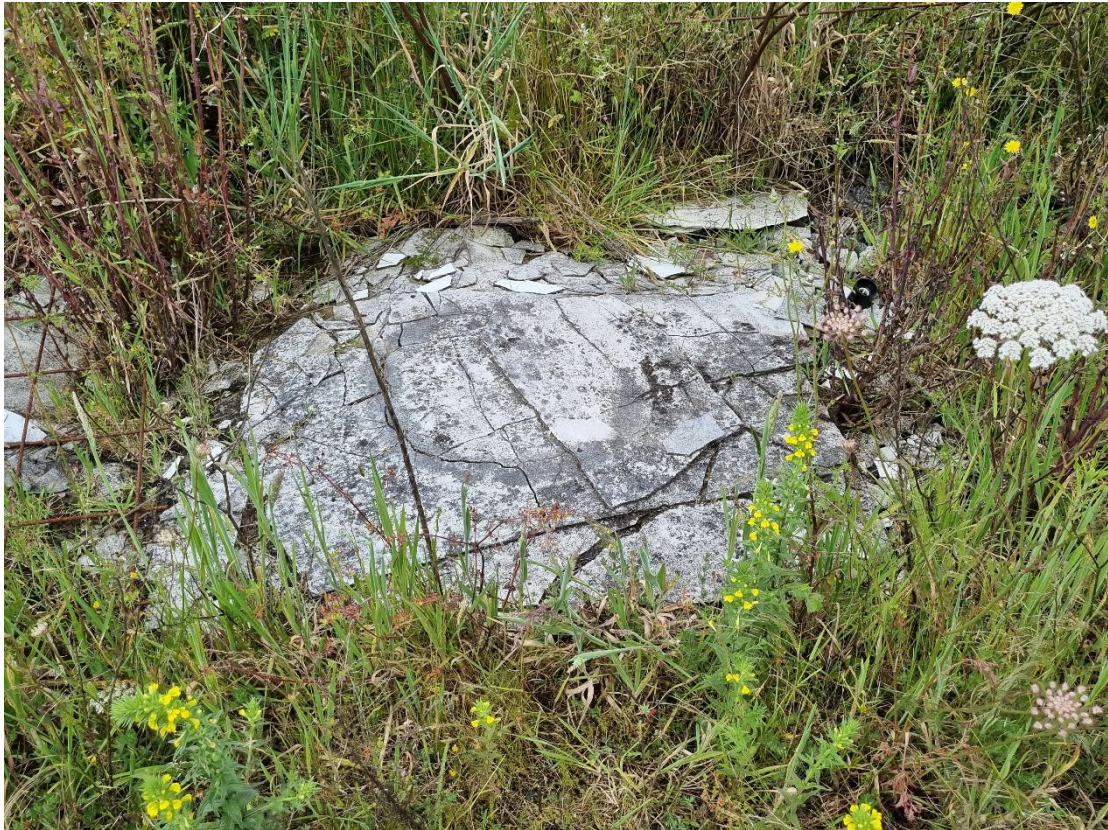
Photograph 7: Broken fibre cement sheets on ground within the unknown yard largely containing shipping containers in the southwest of the site (Feature of interest 5).
