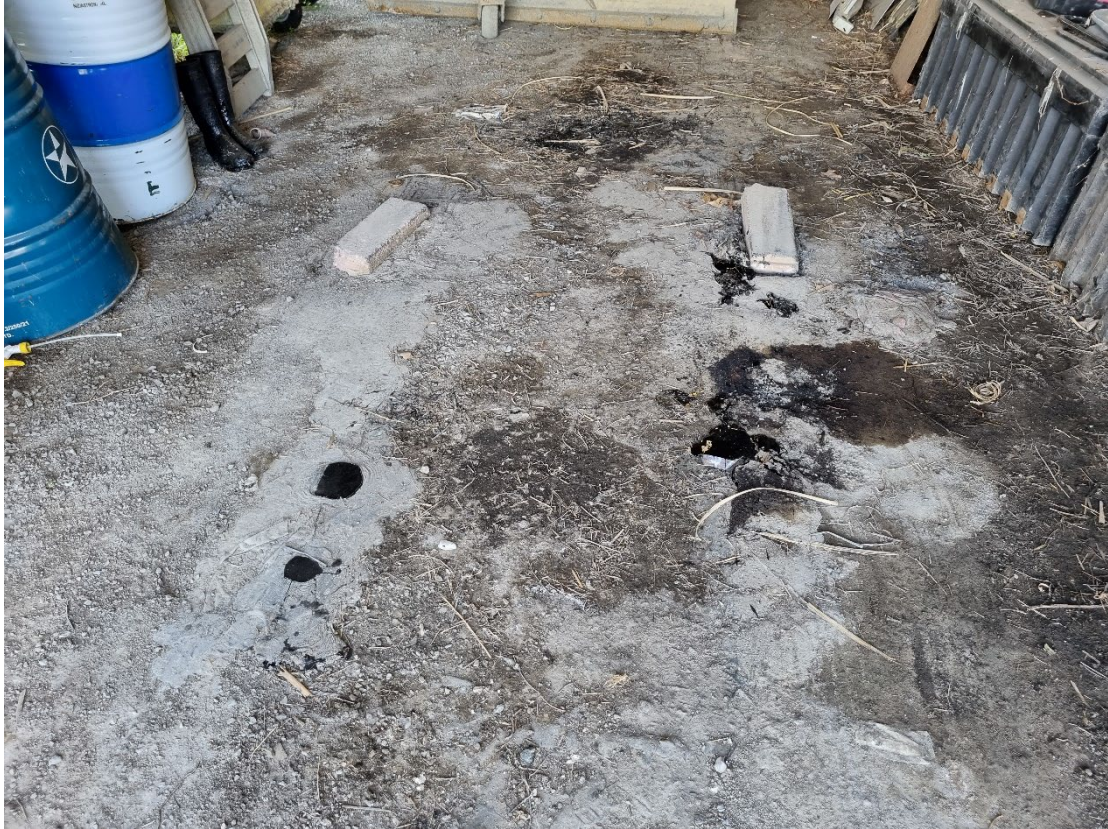
Photograph 21: Example of staining on ground in the 'Workshop'/storage shed (Feature of interest 15).
