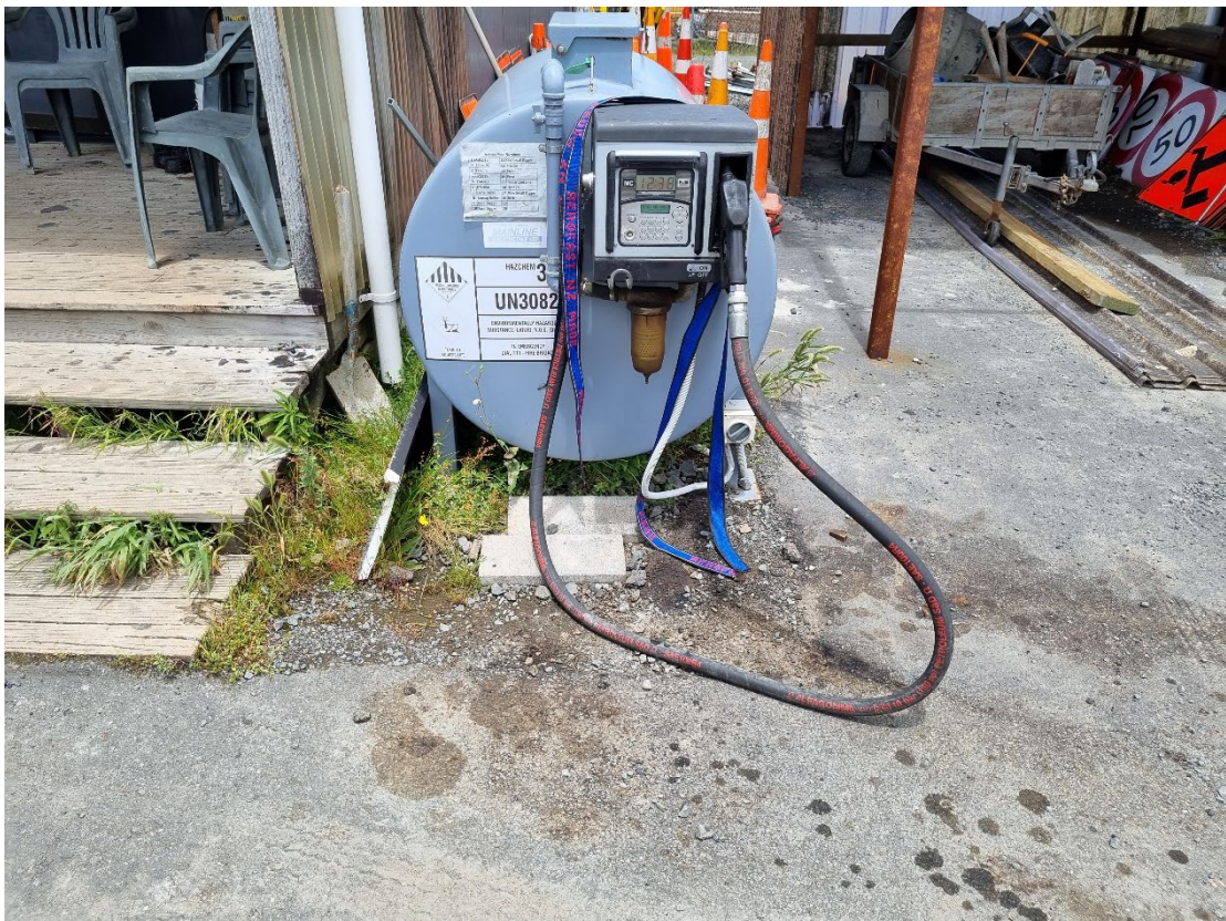
Photograph 16: Un-bunded diesel AST in Shaw Asphalters yard (central north of the site) (Feature of interest 12).
