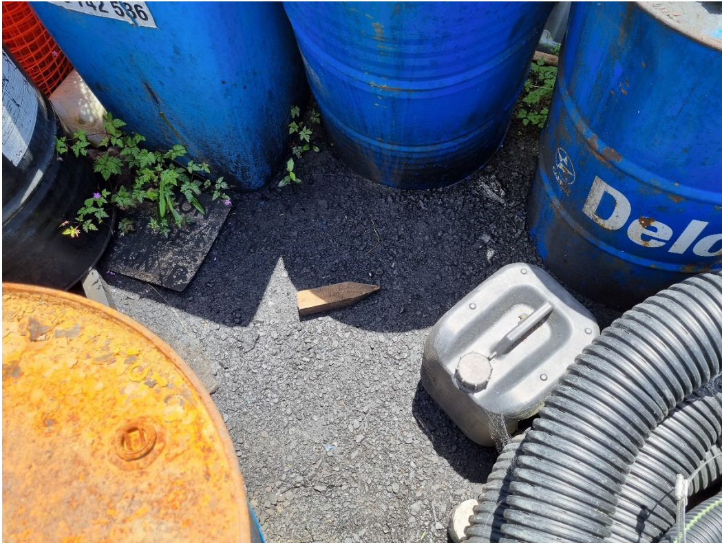
Photograph 19: Stained ground within the 'bund' containing 200L steel drums of kerosene and engine oil behind dangerous goods storage container (Feature of interest 14).
