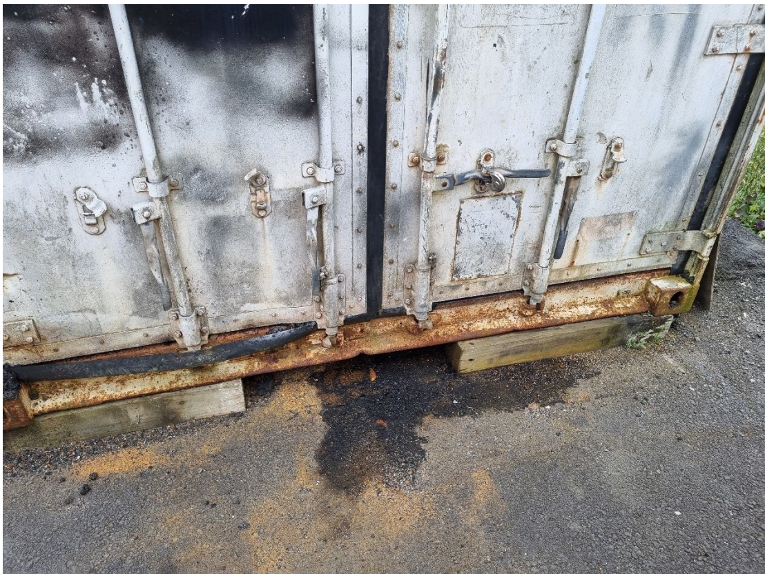
Photograph 2: Staining on asphalt next to locked container in far southeast yard of the site (Feature of interest 1).
