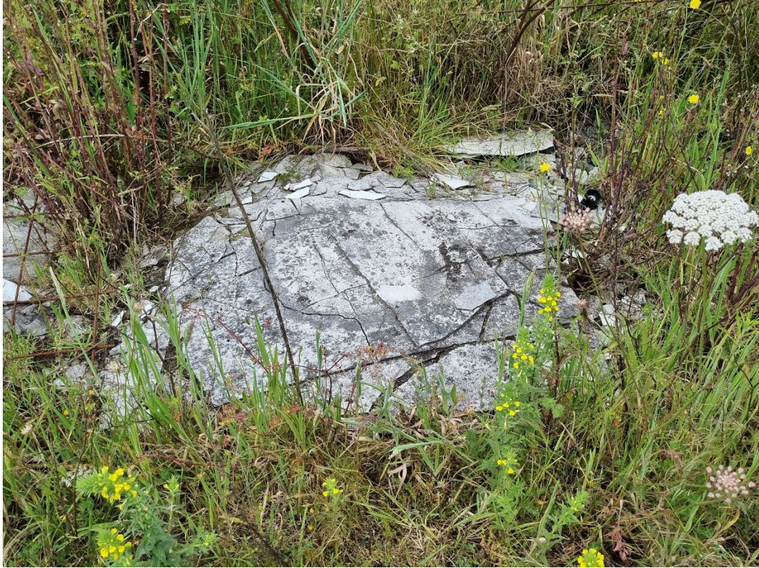
Photograph 7: Broken fibre cement sheets on ground within the unknown yard largely containing shipping containers in the southwest of the site (Feature of interest 5).
