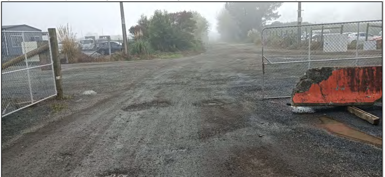
Figure 7: Site visit photo from the entrance of the subject site looking northward down the existing accessway.
