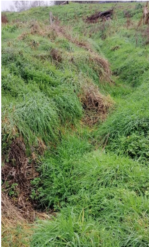
Figure 4: Most of the channel was overgrown with rooted terrestrial vegetation with shallow water.
