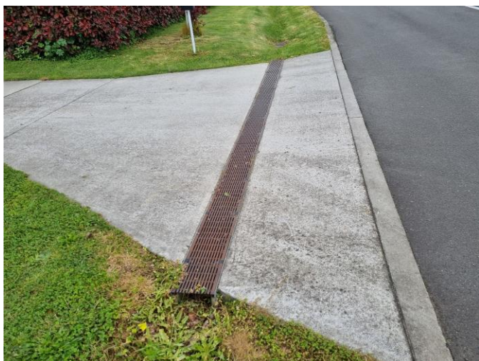
Figure 9: Vehicle crossing slot drain
