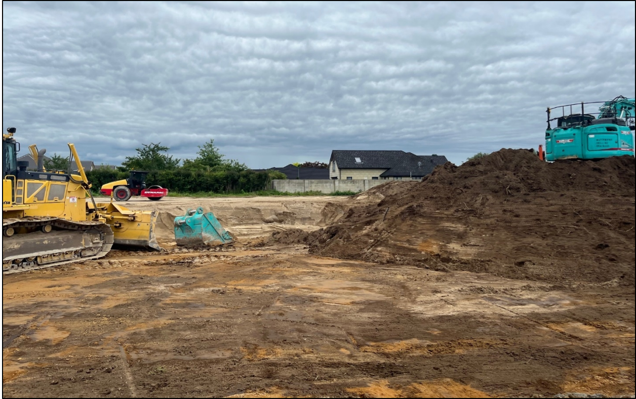
Figure 19: Site visit photo showing area of contaminated site works as consented under LU/0142/23.
